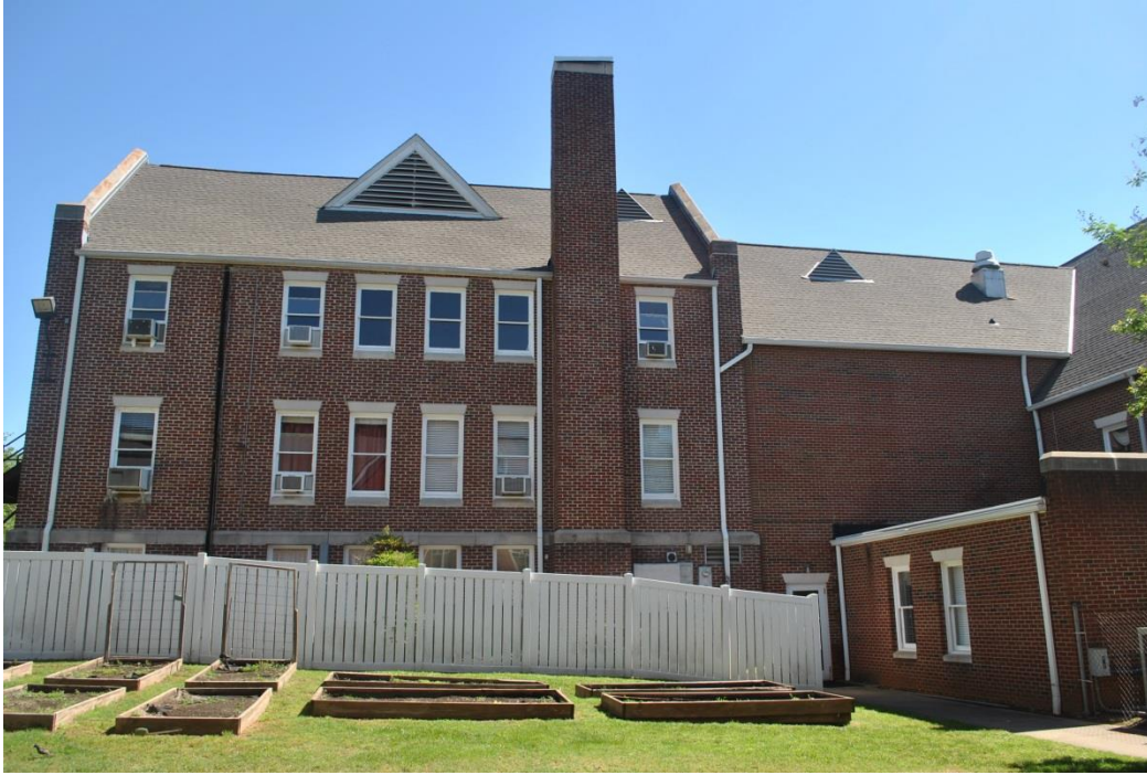
Matthews Presbyterian Church, Rear Classroom Wing, Rear (South) Elevation, and 1976 Classroom Building (Right), Looking Northeast.
